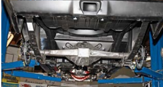
After the leaf springs are installed, the next step is getting the Currie "9+." rear axle housing in place. This is where having lots of friends is a good thing. And here's how it looks. In Part Four, we're going to install the fuel tank, exhaust system, and steering column. It's beginning to look like a car now.
