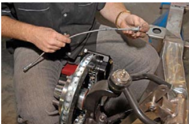
With that done, we see the installation of the provided 3/8-inch, braided stainless brake lines.
