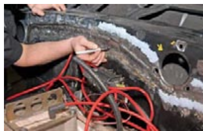
Right off the bat, our installers experienced some clearance issues. For example, the factory GM HEI unit interfered with the Dynacorn Gem's firewall. However, a quick thinking Maxwell realized that an MSD Pro Billet HEI is slightly smaller. A quick substitution immediately rectified the problem.
