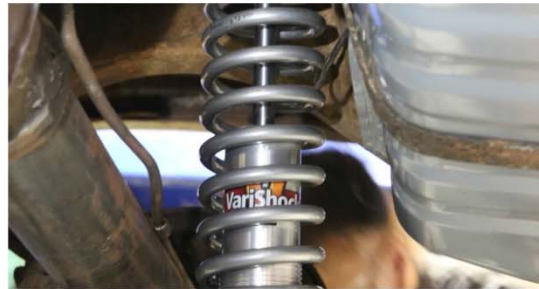
At this point, the install is done and all that is left is putting the weight on the suspension and torquing all the fasteners to spec. The shocks we used are double adjustable, we suggest starting with each setting in the middle of the range and then trial and error adjustments from there to get the ride just how you want it.
